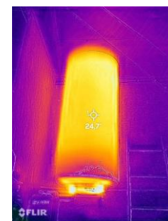
Figure 7: Chauffe-eau non isolé des chevrettes (T=24°C)
