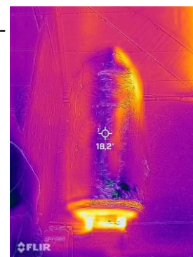
Figure 8: Chauffe-eau isolé des chevrettes (T=18°C)
